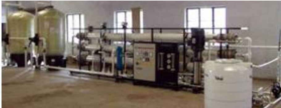
Brackish Water Plant (R.O. System)
