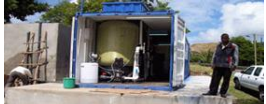
Containerise Brackish Water Plant (R.O. System)
