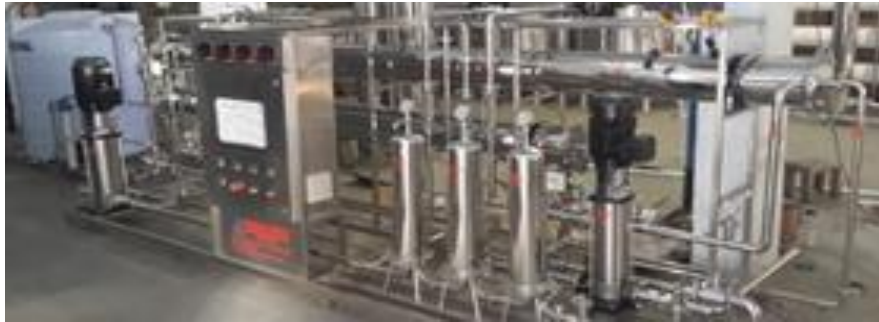
RO System for Pharmaceutical
